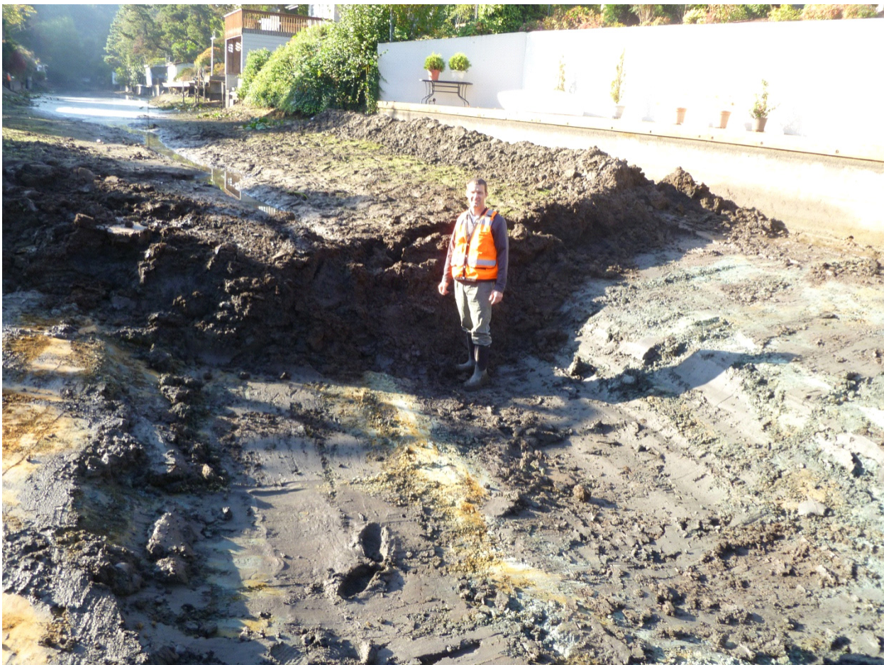
Blue Heron Canal dredge near a storm drain outfall. This sediment accumulated over ten years of storm drain runoff.
